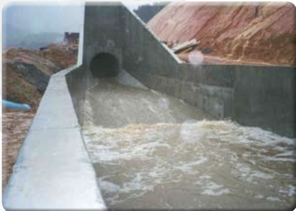
Figure 2. The use of Microsilica 600 for the Wilsons Dam, Upper North Island, NZ reduced permeability and increased resistance to water erosion.
