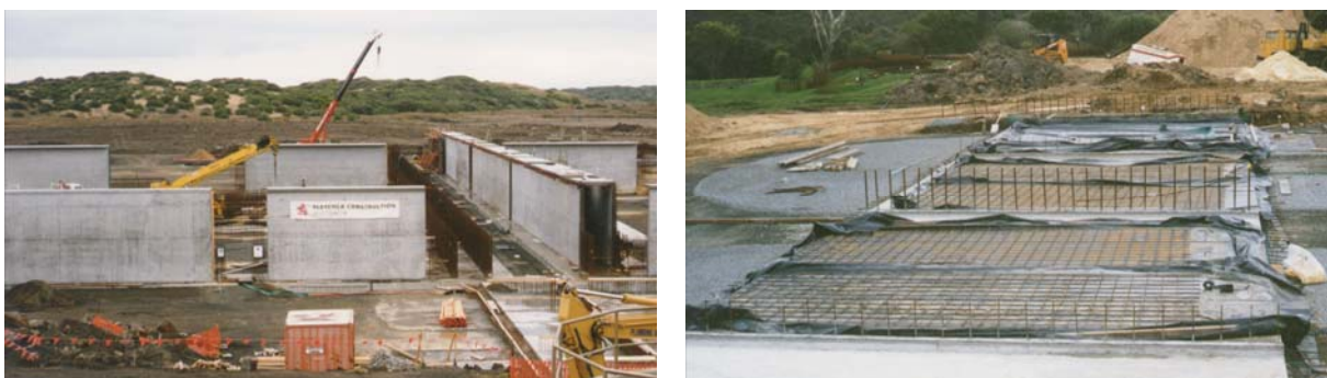
Figure 14 : Black Rock (left) and Anglesea (right) sewage works where Microsilica was used for durability
